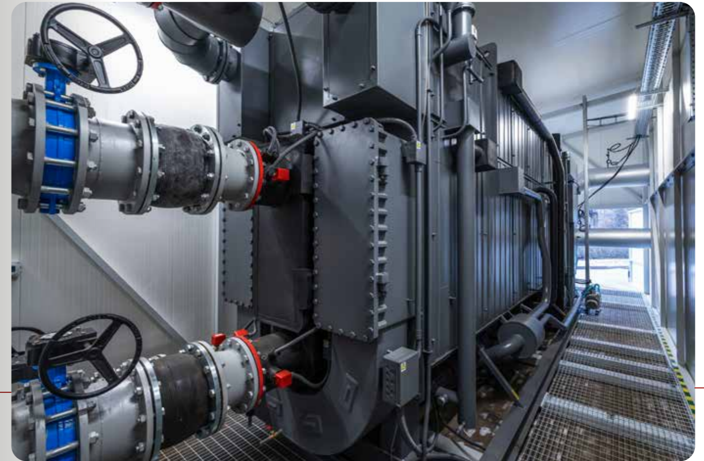
Innovative technology: an absorption heat pump - a step towards decarbonising the heat supply
